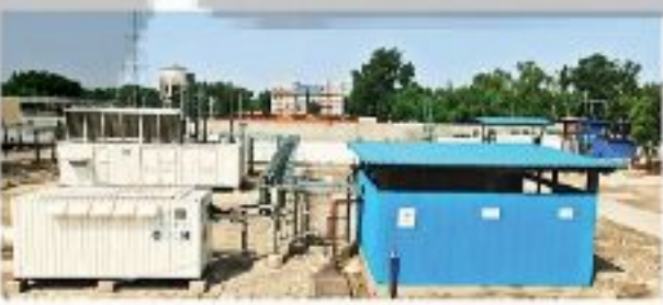
View of Hydrogen Facility
